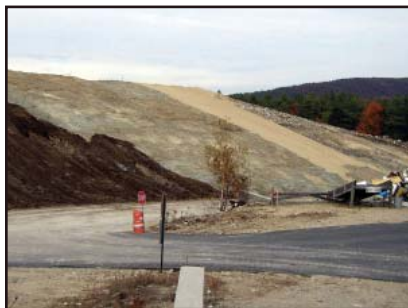
Pulp and paper clay residues (grey) being used to cap a landfill.
